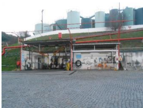
Figura 5.16. Loading Rack Gasóleo
