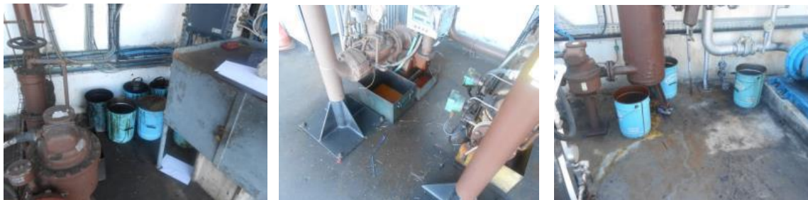
Figura 7.14. Loading Rack Gasóleo
