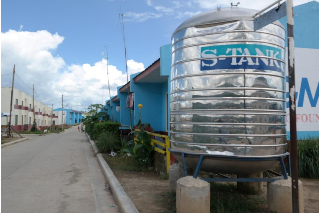
Figure 2.28 - Tacloban North permanent housing water tank (Personal archive, October 2016)
