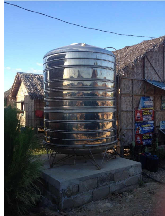
Figure 2.27- Tacloban North temporary shelter water tank (Personal archive, March 2016)
