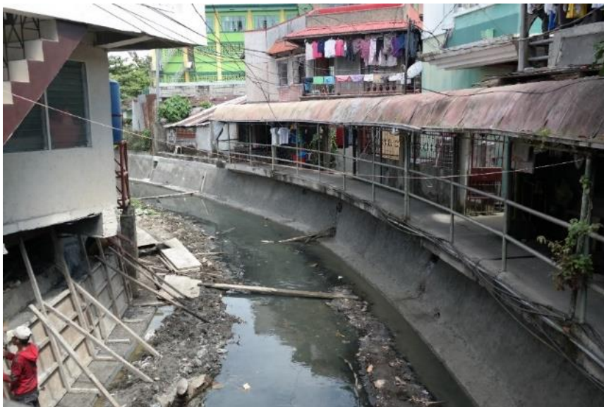
Figure 2.10 - Heavily polluted drainage channel in Tacloban City (Personal archive, March 2016)
