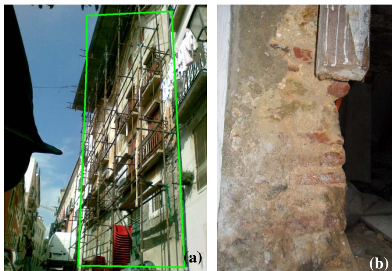
(a) – Fachada; (b) - Pormenor
