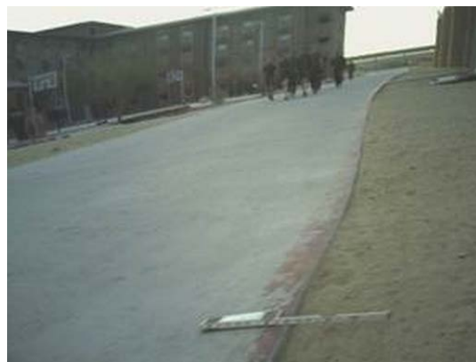
LOW SEVERITY LANE/SHOULDER DROP
