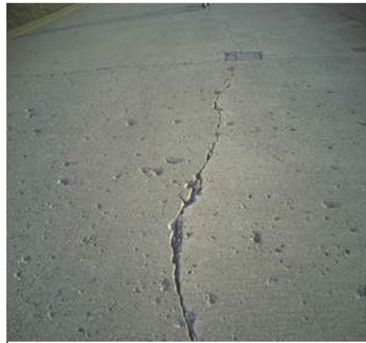
NO SEVERITY LEVEL DEFINED TO POPOUTS
