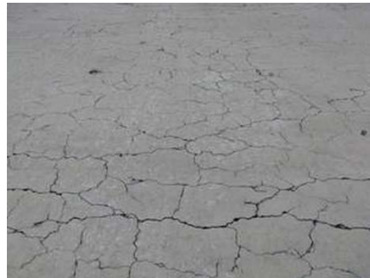
MODERATE SEVERITY LEVEL OF MAP CRACKING AND SCALING
