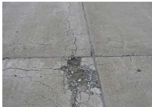
HIGH SEVERITY “D” CRACKING
