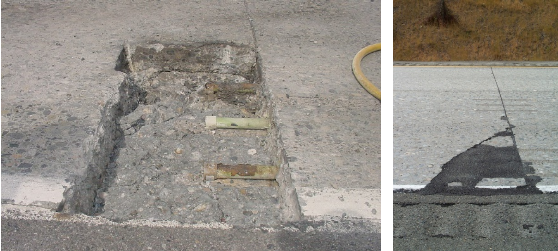
FIGURE 2.10 – EXAMPLE OF A DOWEL BAR CORROSION ON THE LEFT AND ON THE RIGHT A PATCH OVER AN AREA OF DOWEL BAR FAILURE (PAVEMENT INTERACTIVE, 2014 B)
