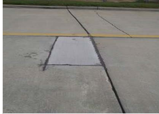
LOW SEVERITY LARGE PATCH
