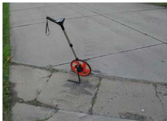
HIGH SEVERITY LARGE PATCH
