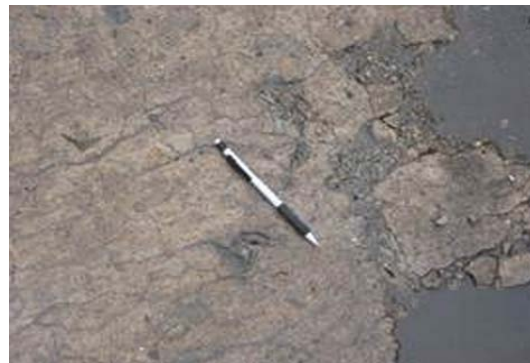
HIGH SEVERITY MAP CRACKING EXAMPLE
