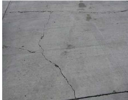
MODERATE SEVERITY SHATTERED SLAB
