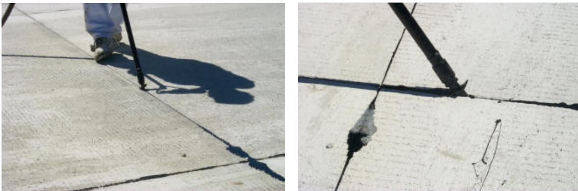
FIGURE 3.1 – ON THE LEFT IS A JOINT SEALING AND IT'S CLOSE-UP ON THE RIGHT (OSU, 2014)
