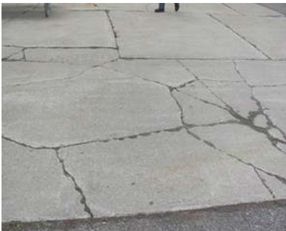
EXAMPLES OF DIVIDED SLAB, LOW, MODERATE AND HIGH SEVERITY LEVELS RESPECTIVELY STARTING IN THE UPPER LEFT FIGURE
