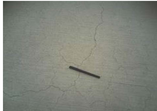
LOW SEVERITY MAP CRACKING EXAMPLE
