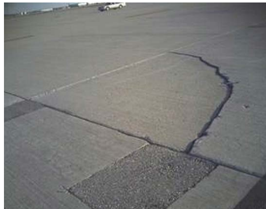
HIGH SEVERITY CORNER BREAK
