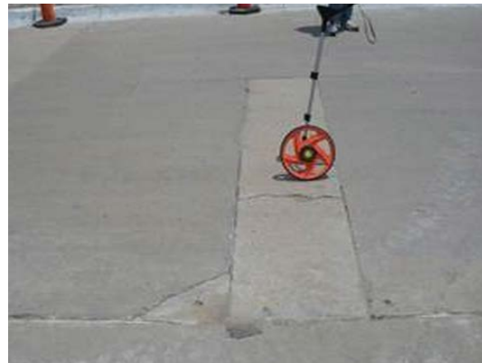
MODERATE SEVERITY LARGE PATCH
