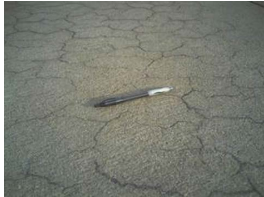
LOW SEVERITY LEVEL OF MAP CRACKING AND SCALING
