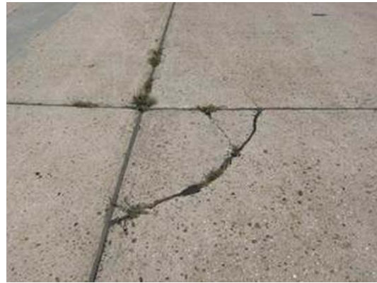
MODERATE SEVERITY CORNER BREAK
