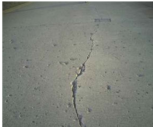
MODERATE SEVERITY L/T/D
