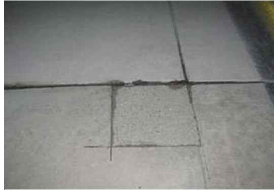
LOW SEVERITY LEVEL OF SMALL PATCHING
