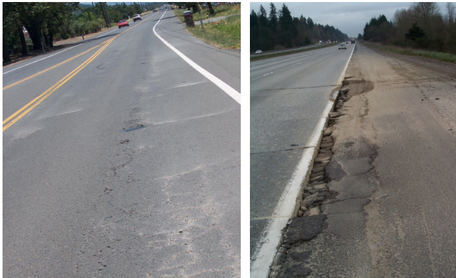
FIGURE 2.19 – ON THE LEFT IT’S AN EXAMPLE OF PUMPING IN ACTION AND ON THE RIGHT IS AN EXAMPLE OF PUMPING DISTRESS (PAVEMENT INTERACTIVE, 2014 B)
