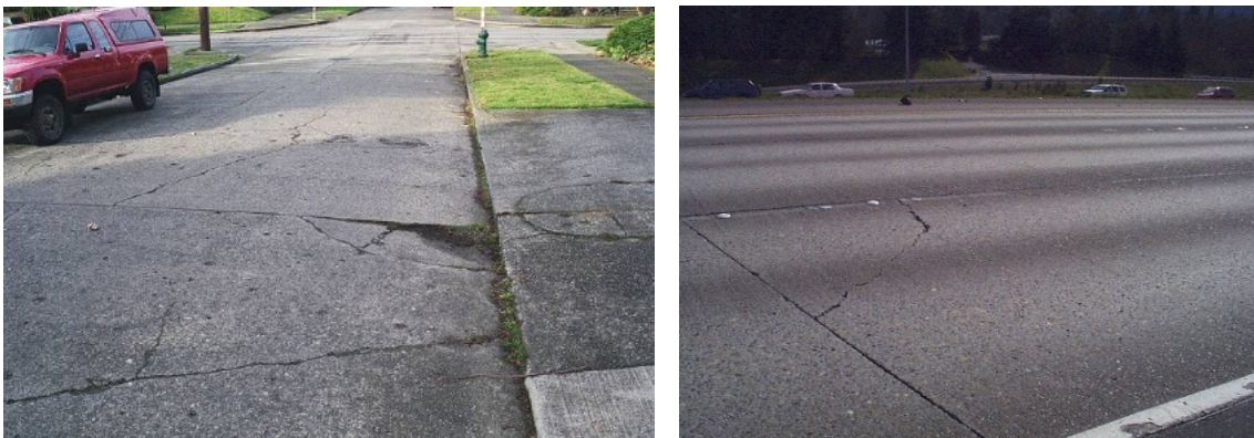
FIGURE 2.7 – EXAMPLES OF CORNER BREAKS AT A HIGH VOLUME TRAFFIC ROAD (PAVEMENT INTERACTIVE, 2014 B)
