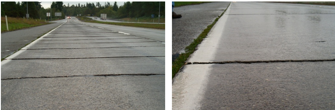
FIGURE 2.20 – EXAMPLE OF FAULTING DISTRESS AT THE LEFT AND A CLOSE-UP ON THE RIGHT ( PAVEMENT INTERACTIVE, 2014 B)
