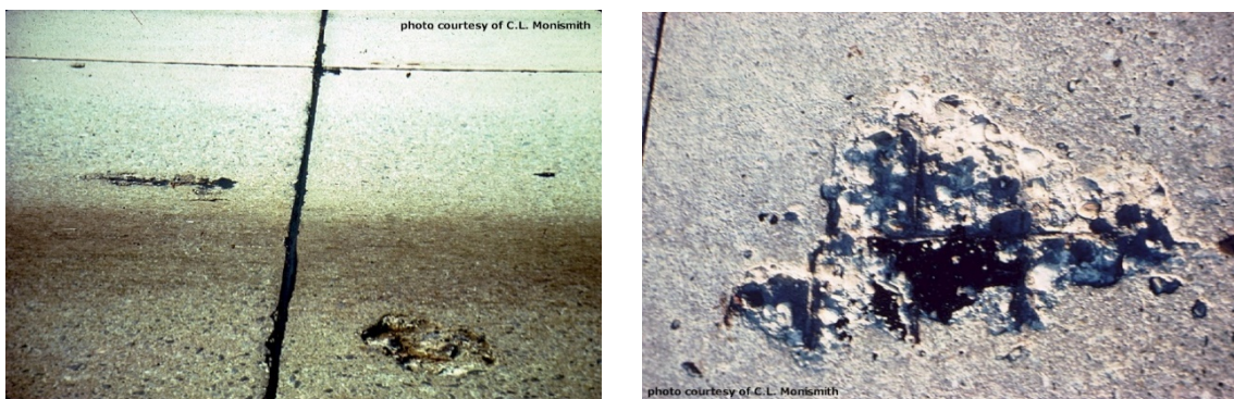
FIGURE 2.17 – EXAMPLES OF POPOUTS DISTRESS (PAVEMENT INTERACTIVE, 2014 B)
