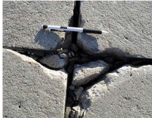
HIGH SEVERITY CORNER SPALLING
