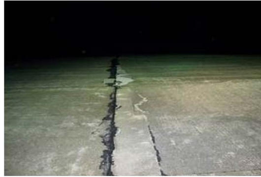
LOW SEVERITY LEVEL OF BLOWUPS
