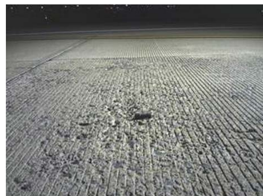
HIGH SEVERITY LEVELS OF MAP CRACKING AND SCALING
