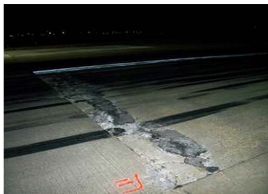
HIGH SEVERITY LEVEL OF BLOWUPS
