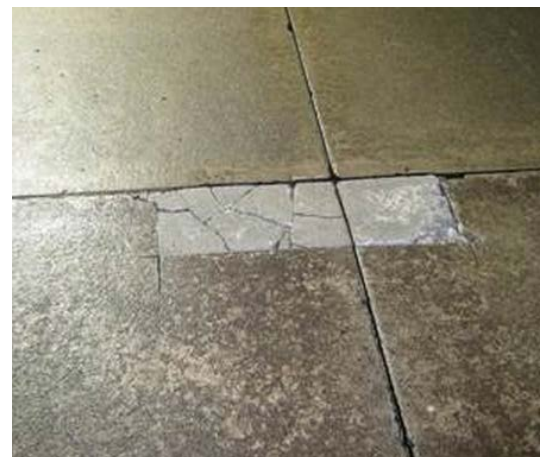
LOW SEVERITY LEVEL OF SMALL PATCHING
