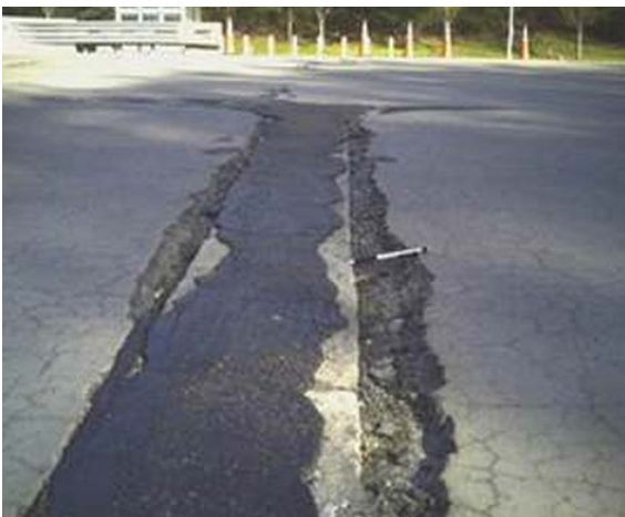
EXAMPLES OF JOINT SPALLING DISTRESS ON ROADS, FROM LEFT TO RIGHT, LOW, MODERATE AND HIGH SEVERITY LEVELS RESPECTIVELY
