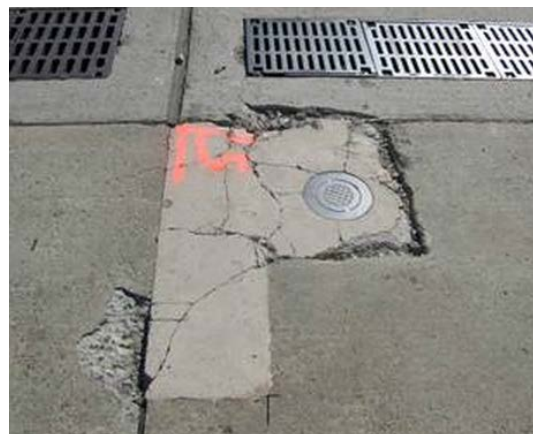
HIGH SEVERITY LEVEL OF LARGE PATCHING
