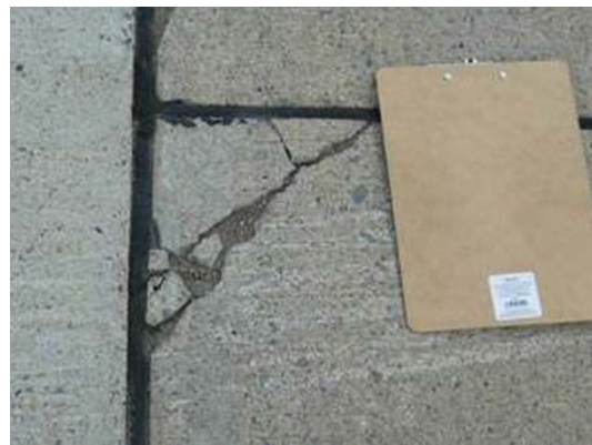
MODERATE SEVERITY CORNER SPALLING
