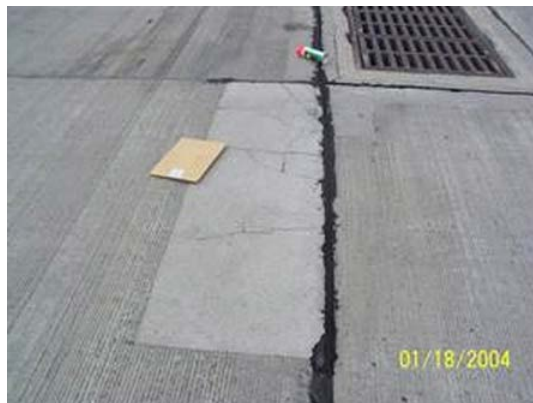
MODERATE SEVERITY LEVEL OF LARGE PATCHING
