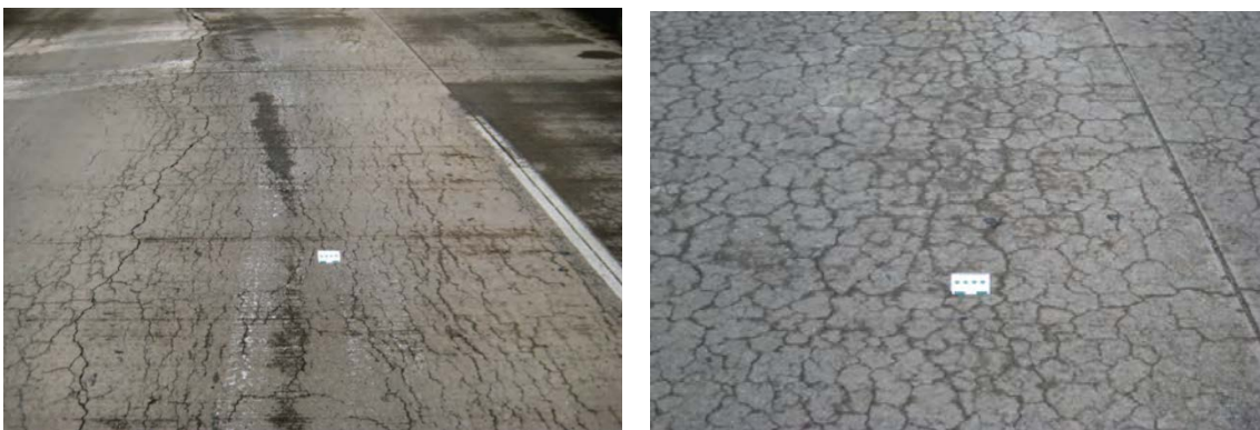
FIGURE 2.12 – EXAMPLES OF MAP CRACKING RESULTING FROM ALKALI-AGGREGATE REACTION (THOMAS, FOURNIER, FOLLIARD, & RESENDEZ, 2011)
