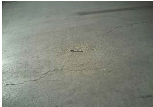
MODERATE SEVERITY MAP CRACKING EXAMPLE
