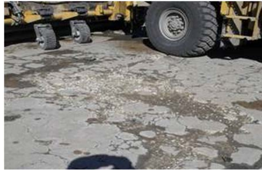
HIGH SEVERITY LEVEL OF ASR
