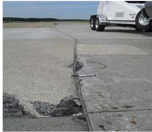
HIGH SEVERITY LEVEL OF BLOWUPS
