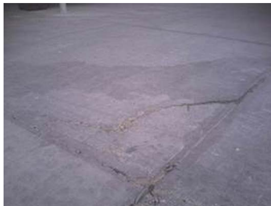
EXAMPLE OF HIGH SEVERITY CORNER BREAK
