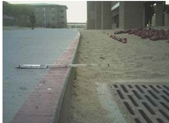
HIGH SEVERITY LANE/SHOULDER DROP
