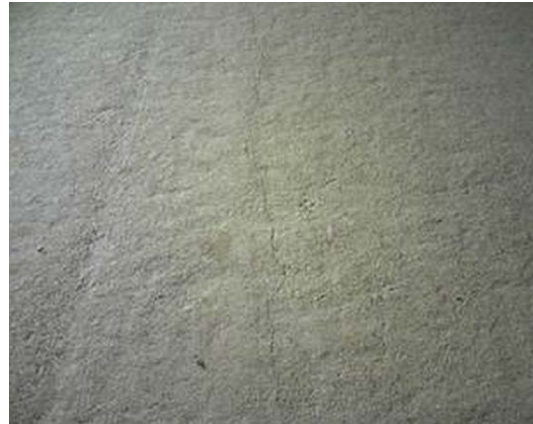
NO SEVERITY LEVELS DEFINED TO SHRINKAGE CRACKING
