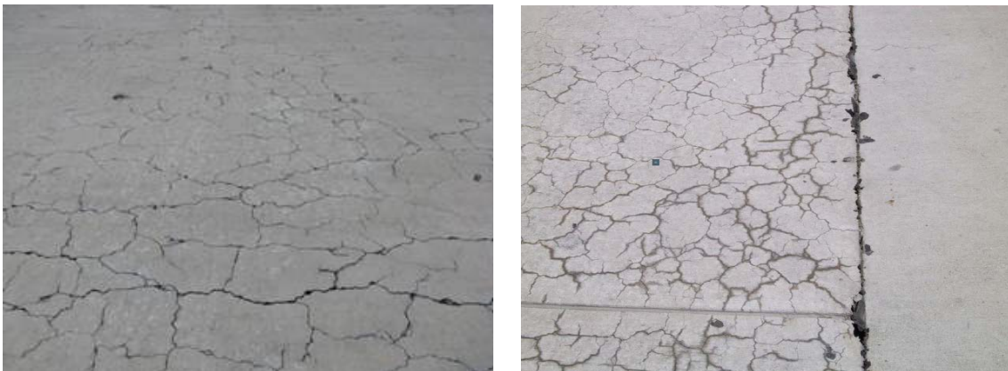
FIGURE 5.7 – ON THE LEFT THERE IS AN EXAMPLE OF SCALING/MAP CRACKING AND ON THE RIGHT AN EXAMPLE OF ASR WITH JOINT SEALANT FAILURE (THOMAS, FOURNIER, FOLLIARD, & RESENDEZ, 2012)
