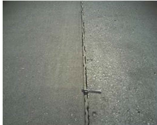
MODERATE SEVERITY LEVEL JOINT SEAL DAMAGE
