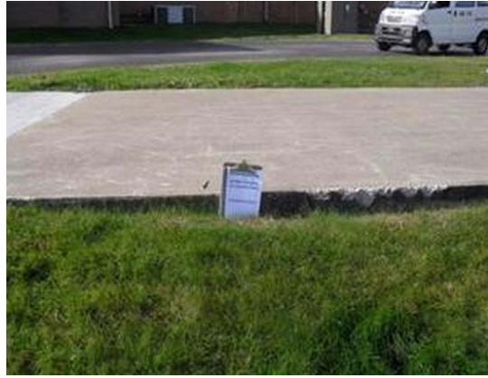
MODERATE SEVERITY LANE/SHOULDER DROP.
