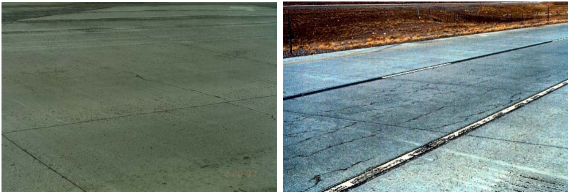
FIGURE 2.8 – EXAMPLE OF SHRINKAGE CRACKING ON NEW SLABS ON THE LEFT AND SEVERE SHRINKAGE CRACKING ON THE RIGHT (PAVEMENT INTERACTIVE, 2014 B)
