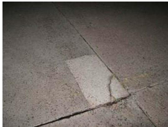
MODERATE SEVERITY LEVEL OF SMALL PATCHING
