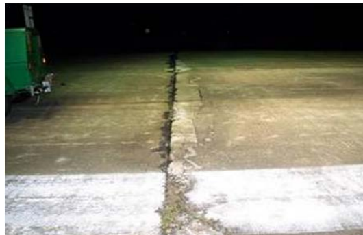
MODERATE SEVERITY LEVEL OF BLOWUPS
