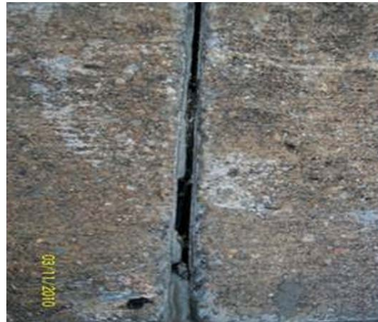
HIGH SEVERITY LEVEL JOINT SEAL DAMAGE
