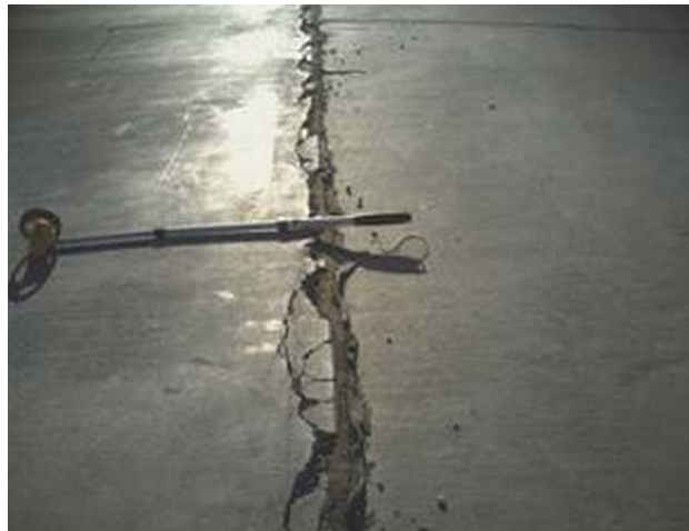
EXAMPLE OF FAULTING
