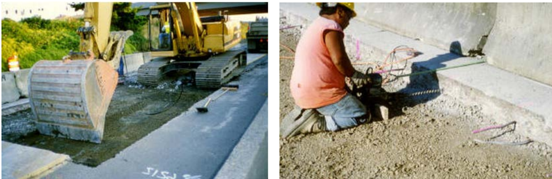
FIGURE 3.5 – ON THE LEFT IS A BASE PREPARATION TO FULL DEPTH PATCH AND ON THE RIGHT IS A WORKER DRILLING HOLES FOR A TIE BAR PLACEMENT (OSU, 2014)
