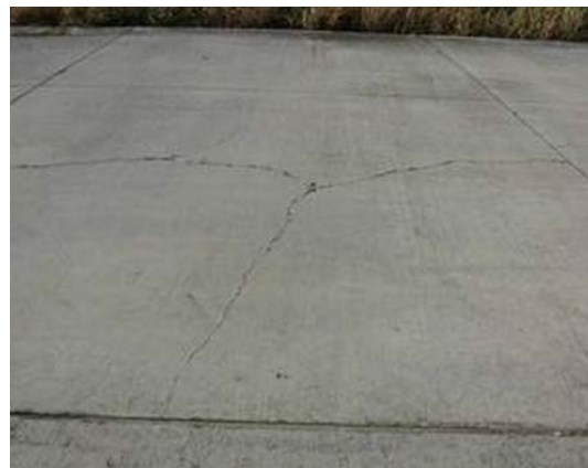
LOW SEVERITY SHATTERED SLAB
