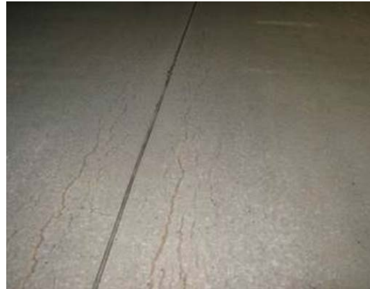
LOW SEVERITY “D” CRACKING
