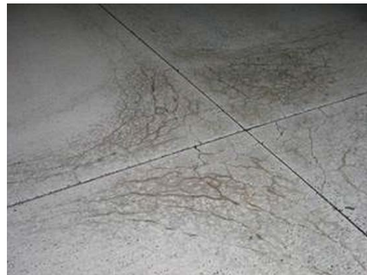
MODERATE SEVERITY “D” CRACKING
