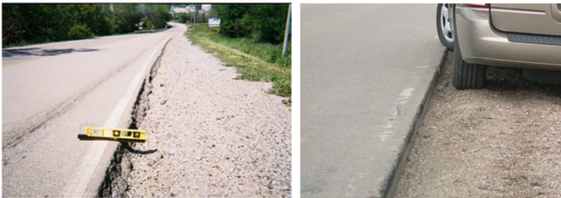
FIGURE 2.22 – EXAMPLES OF LANE/SHOULDER DROPOFF (FHA, 2014 B)
