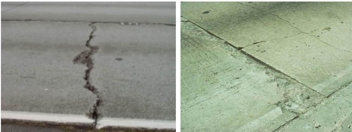
FIGURE 2.13 – EXAMPLES OF SPALLING ALONG A LINEAR CRACK ON THE LEFT (PAVEMENT INTERACTIVE, 2014 B) AND A JOINT AND CORNER SPALLING ON THE RIGHT (FLORIDA DEPARTMENT OF TRANSPORTATION, 2012)
