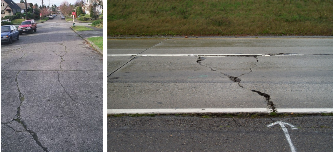
FIGURE 2.5 – EXAMPLES OF LONGITUDINAL AND DIAGONAL CRACKS ON THE LEFT AND ON THE RIGHT TRANSVERSE AND DIAGONAL CRACKS (PAVEMENT INTERACTIVE, 2014 B)
