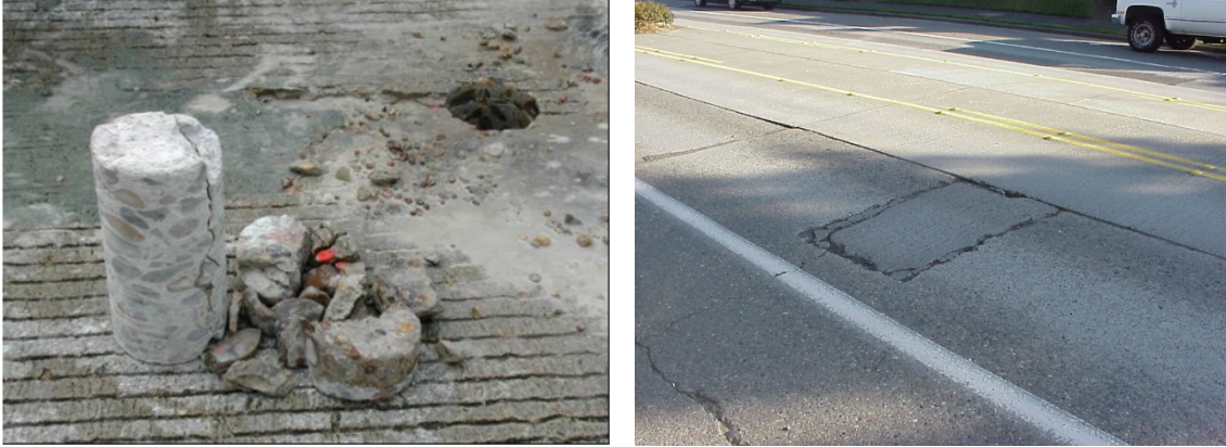
FIGURE 3.4 – CORING FROM SPALL REPAIRED AREA ON THE LEFT AND ON THE RIGHT A SMALL PATCH EXAMPLE (PAVEMENT INTERACTIVE, 2014 C)
