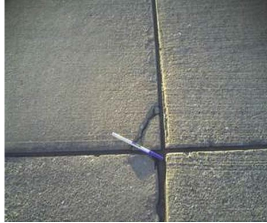
LOW SEVERITY CORNER SPALLING
