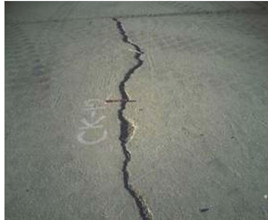
HIGH SEVERITY CRACK AT A ROAD
