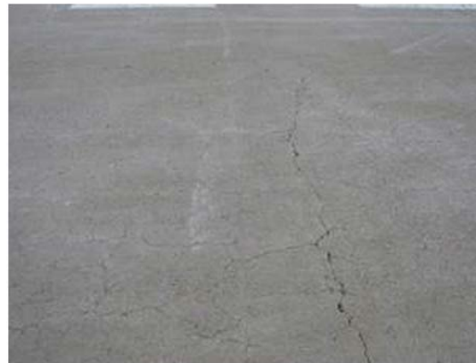
LOW SEVERITY LEVEL OF ASR
