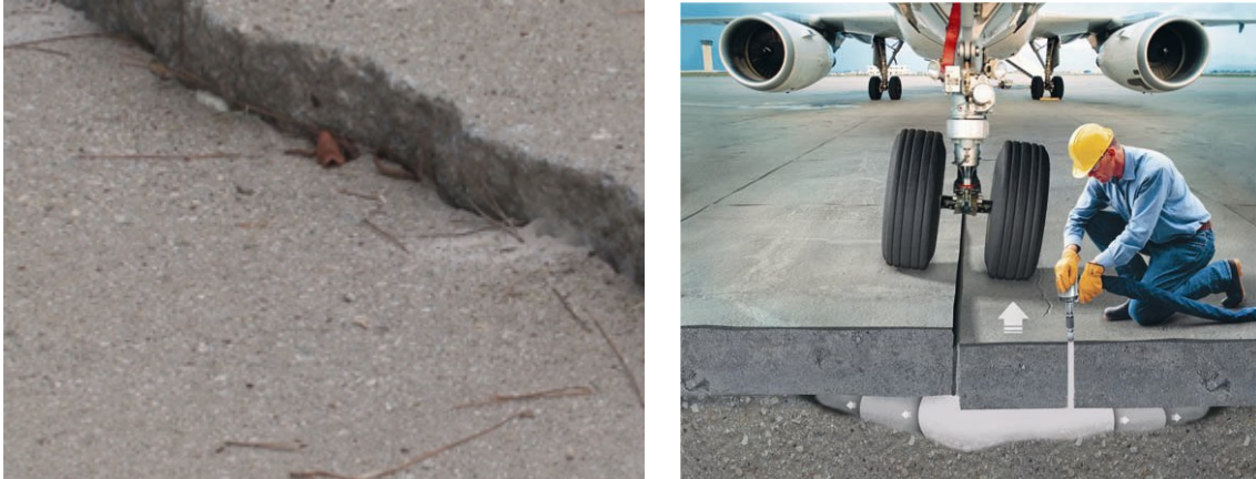
FIGURE 3.2 – DIFFERENCE OF ELEVATION DUE TO PUMPING, CONSOLIDATION OR OTHER MEANS ON THE LEFT (PRIME RESINS, 2014) AND AN EXAMPLE OF SLAB STABILIZATION ON THE RIGHT (EAGLE LIFTING, 2014)
