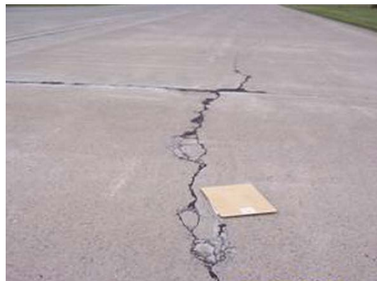
HIGH SEVERITY L/T/D
