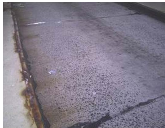
EXAMPLE OF MAP CRACKING AND SCALING DISTRESS
