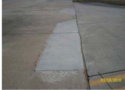
LOW SEVERITY LEVEL OF LARGE PATCHING
