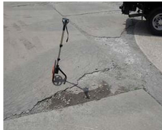
HIGH SEVERITY DURABILITY CRACKING
