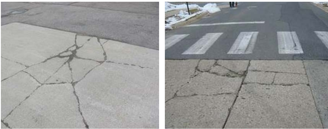
EXAMPLES OF PUNCHOUT DISTRESS AT HIGH SEVERITY
