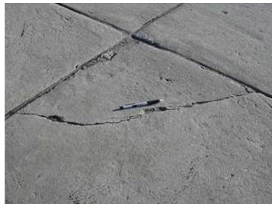
LOW SEVERITY CORNER BREAK
