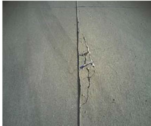
MODERATE SEVERITY LEVEL OF SPALLING L/T JOINTS
