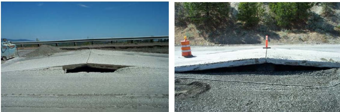
FIGURE 2.14 – EXAMPLES OF BLOWUP DISTRESS (PAVEMENT INTERACTIVE, 2014 B)
