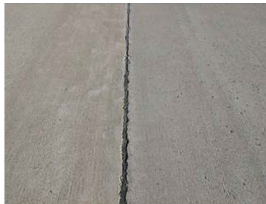
LOW SEVERITY LEVEL JOINT SEAL DAMAGE
