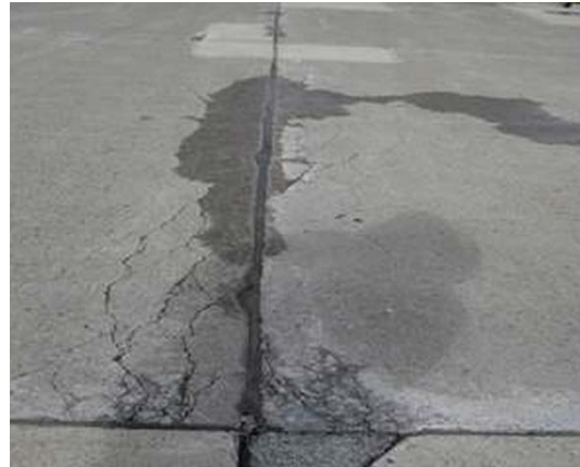
MODERATE DURABILITY CRACKING
