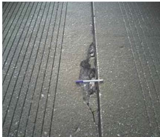
HIGH SEVERITY LEVEL OF SPALLING L/T JOINTS
