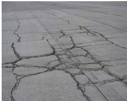
HIGH SEVERITY SHATTERED SLAB
