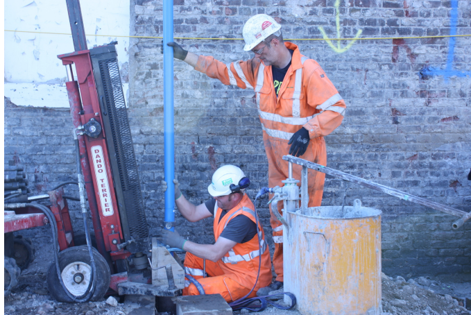
Figure 2.1: Installation of an inclinometer casing in the ground of a work site [16]
