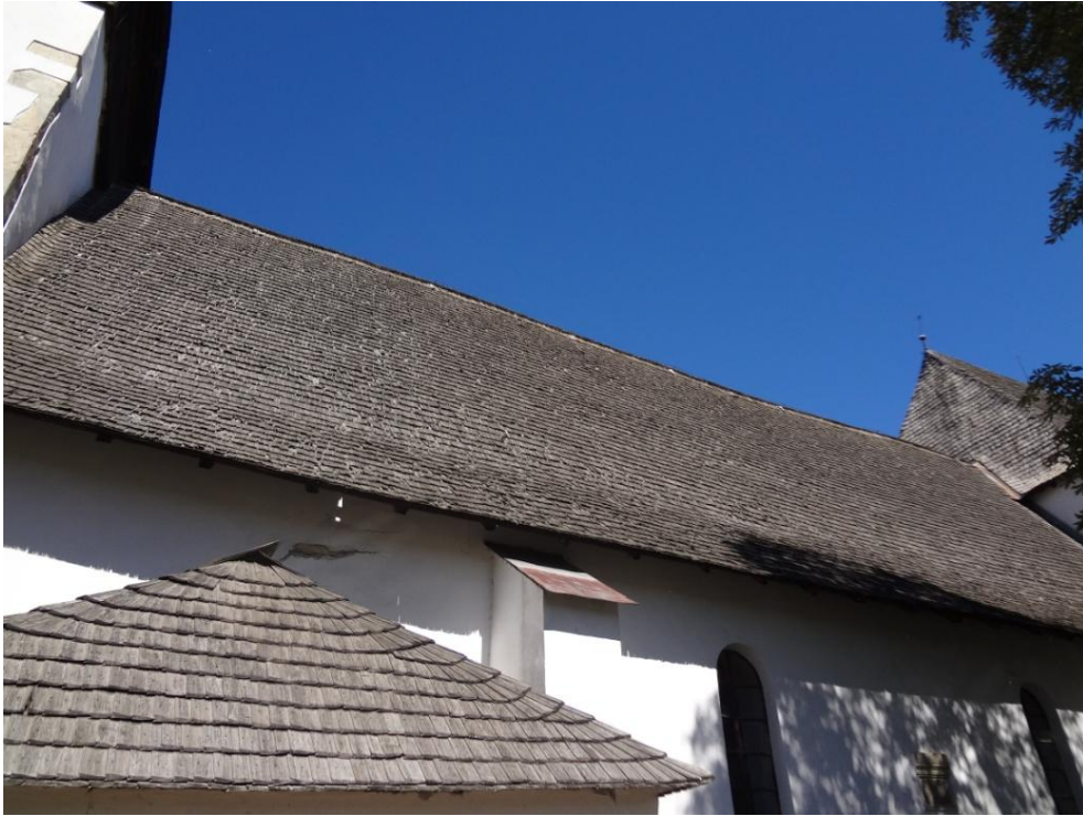
Fig. 4.17 – Shingles in bad condition.
