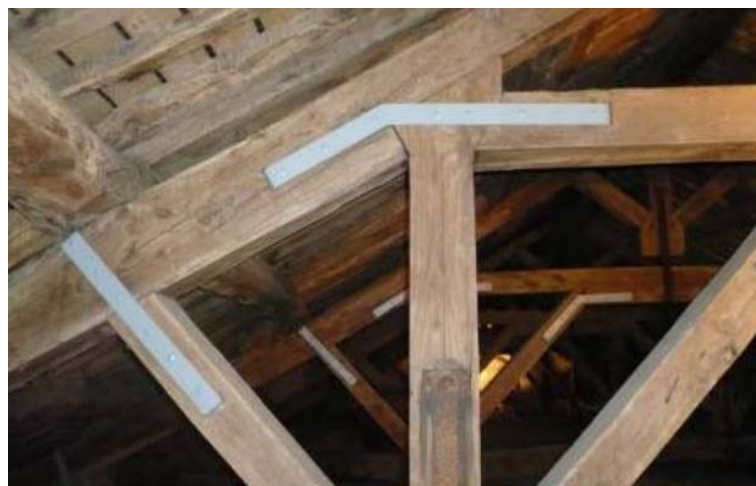
Fig. 3.36 – Use of traditional steel elements to improve the connection between timber elements [37].
