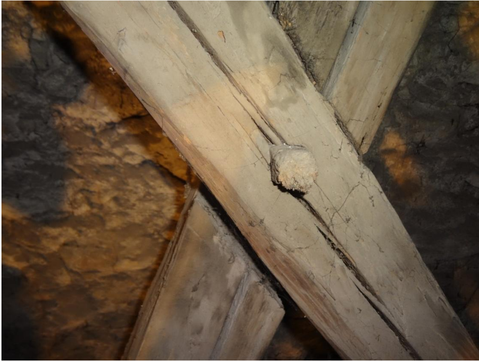
Fig. 4.23 – Longitudinal cracks in the structural elements.
