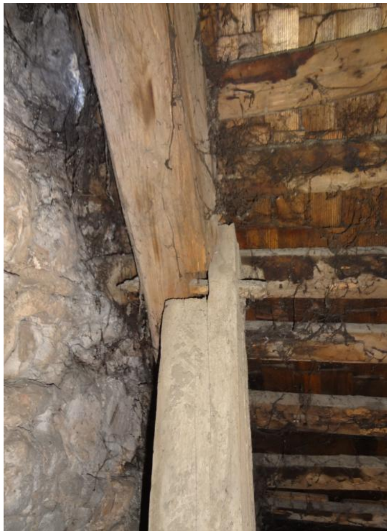
Fig. 4.24 – Gap between rafter and angle brace.
