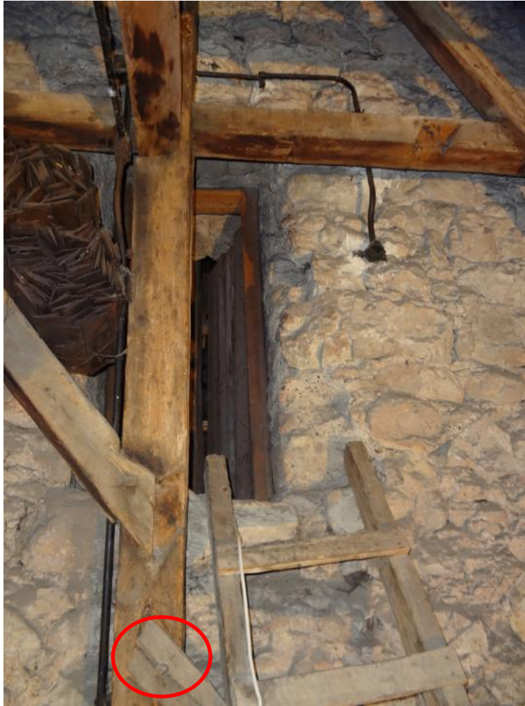
Fig. 4.15 – Missing upper knee brace and deteriorated angle brace connection.
