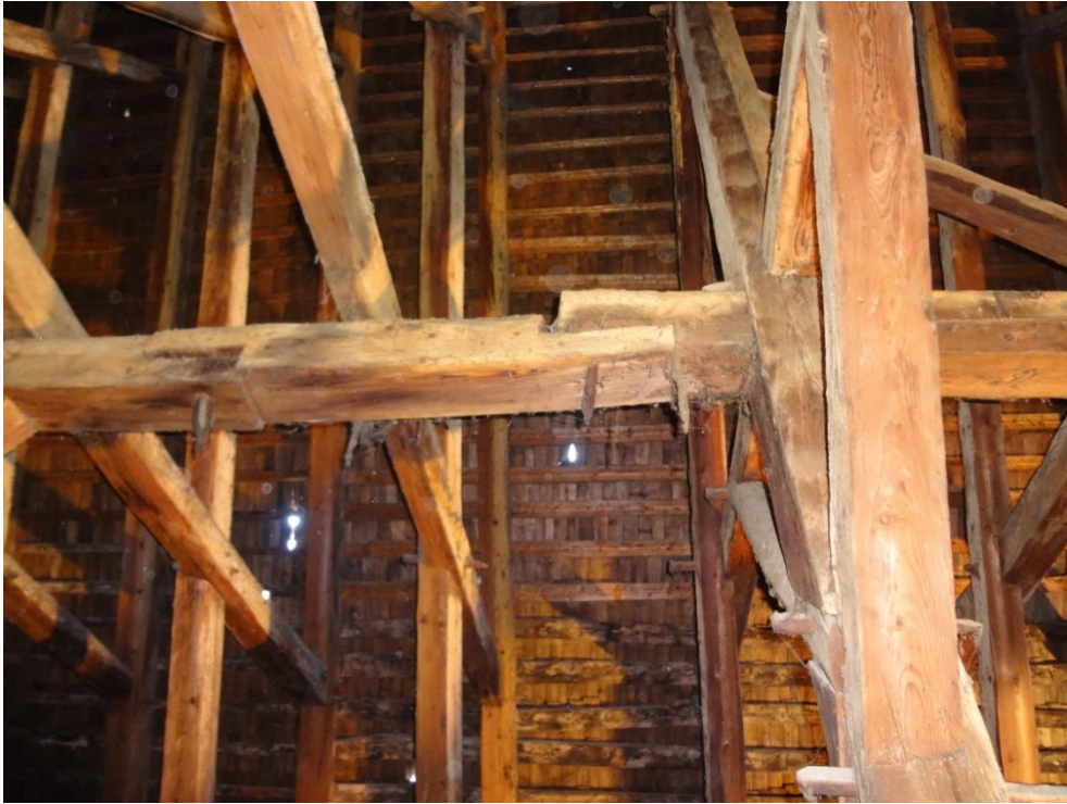
Fig. 4.25 – Gap in upper plate extension joint.
