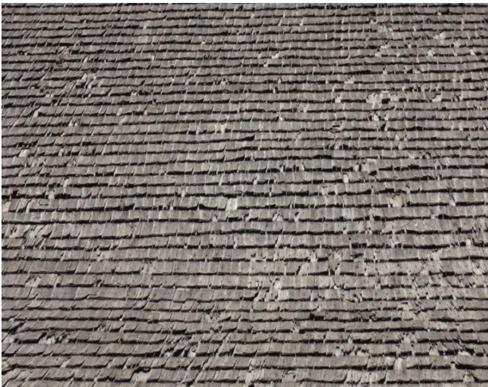
Fig. 4.18 – Shingles in bad condition – detail.
