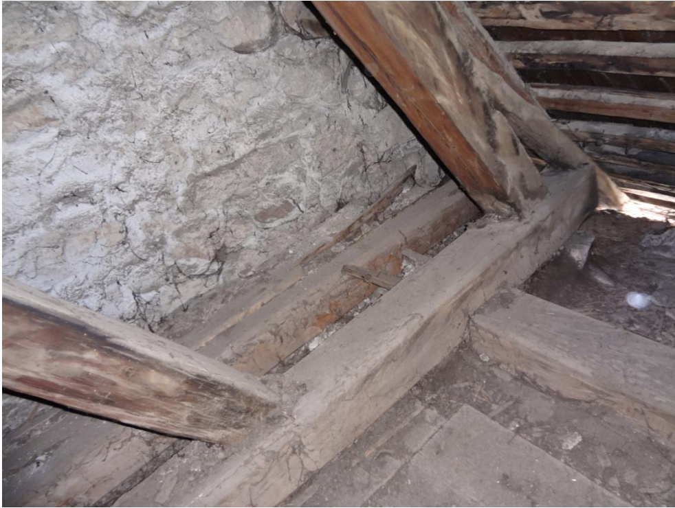
Fig. 4.21 - Both tie beams are deteriorated in the first truss, especially in the extremities.
