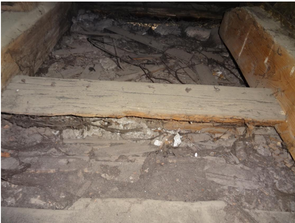
Fig. 4.16 – Deteriorated wall plate.
