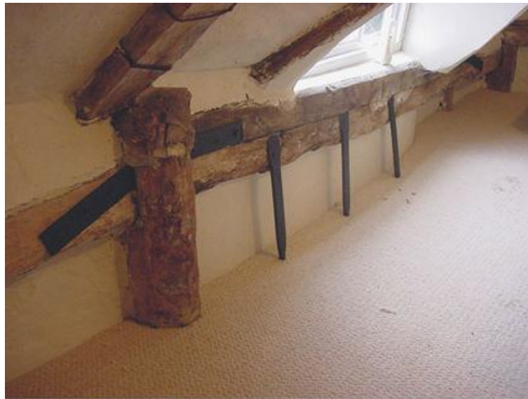
Fig. 3.7 – Copious ironwork was amateurishly inserted to arrest its collapsing floors and splaying walls [3].
