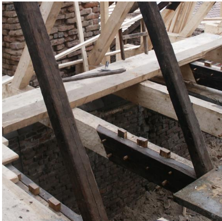
Fig. 3.28 – Old – new timber to timber connection.
