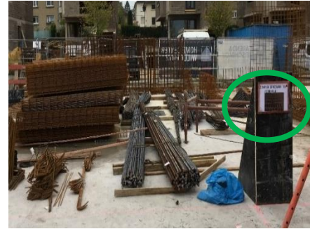
Figure 7: Example of a 5S stockage area
