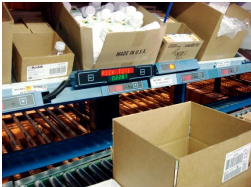
Figura 2.11. Sistema Picking-to-light , da marca Sickinsight.
