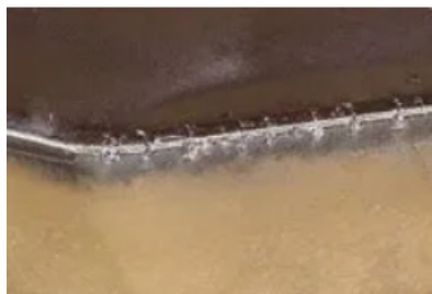
Figure 2.21: Thermal cracks - Example [41]
