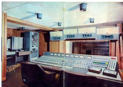
Photo 15 - Control room, upper floor with the four monitors in front of the console (photo courtesy of José Manuel Fortes)
