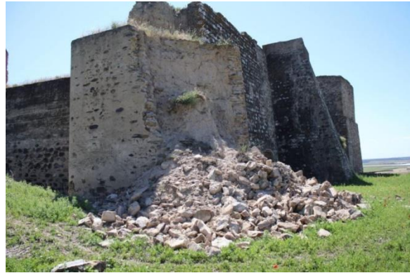
Figure 3.2: Tower of Juromenha Castle that collapsed in 2008 (source (Dias 2018)).
