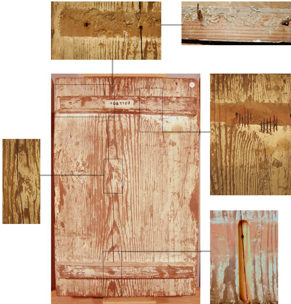
Figure 29. Wood interventions and crack detail
