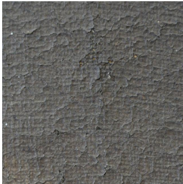
Figure 2.12: Detail of the mechanical cracks.
