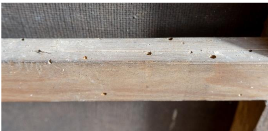
Figure 2.4: Xylophagous insect exit holes on the horizontal crossbar.
