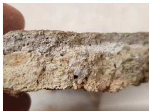
Figure 26. Sample of the render of the East façade with a cementitious repair coat.
