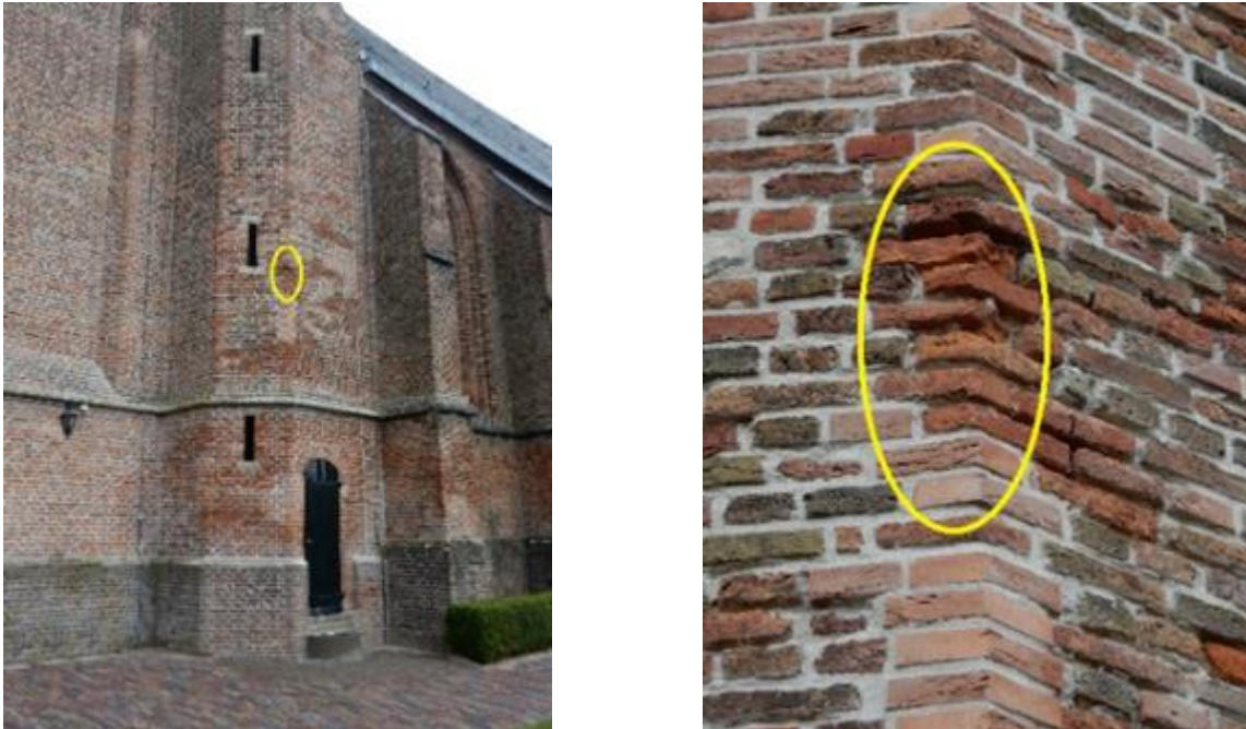
Figure 21. Situation of the damage in 2016. Left, the reddish parts of the masonry indicate where the repointing is damaged. Right, detail of one of the spots with damaged repointing.
