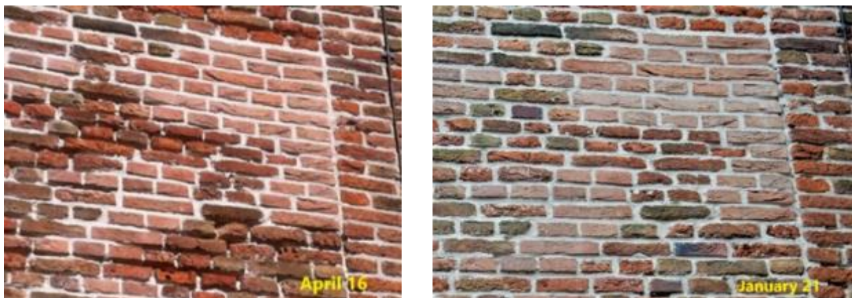
Figure 22. Comparison of part of the south wall in April 2016 (before repair), respectively January 2021. Most of the underburnt bricks are still in place (some of the weakest were replaced). The repair repointing performs rather satisfactorily.
