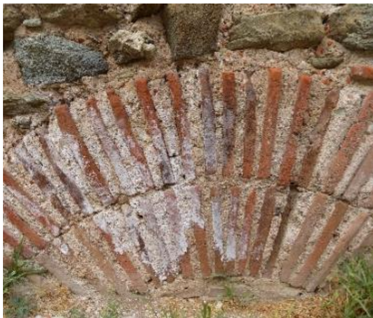
Figure 31. Efflorescence near to the ground level.
