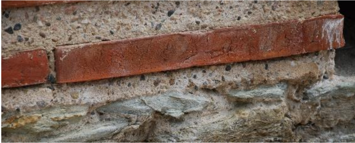
Figure 30. Repair mortar in a mix structural system of Galerius Palace in Thessaloniki, Greece.
