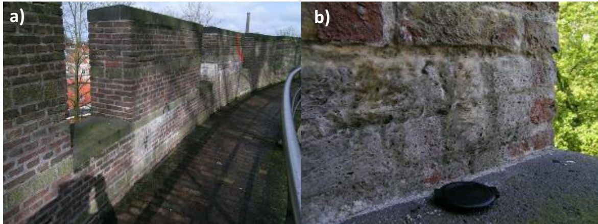
Figure 32. a) Encrustation, due to leaching of mortar in very exposed masonry, the battlements of a motte castle; b) Detail.
