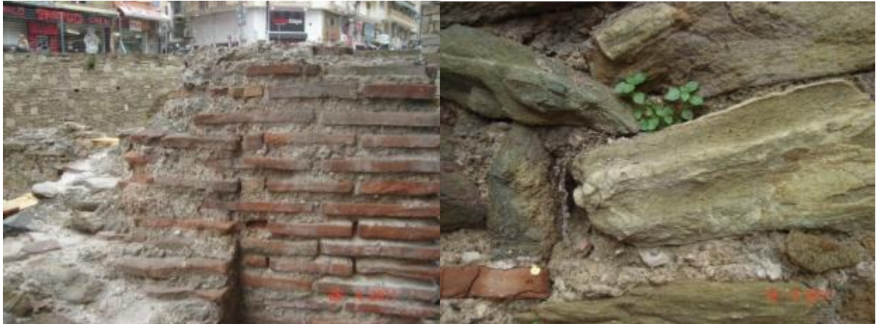
Figure 29. Deterioration problems of the masonries before the intervention works.
