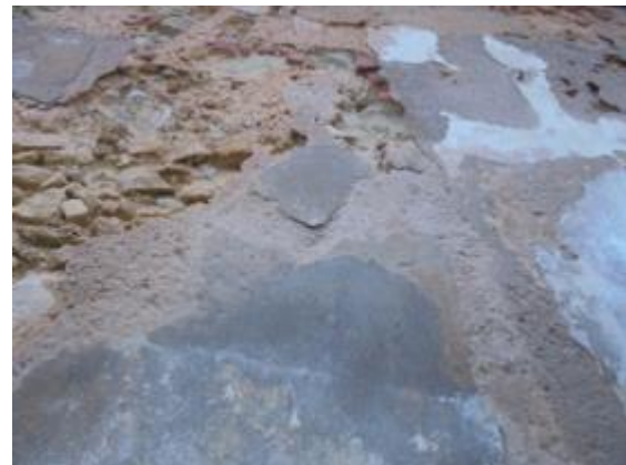
Figure 24. Detail of the degradation showing cementitious repair mortars.
