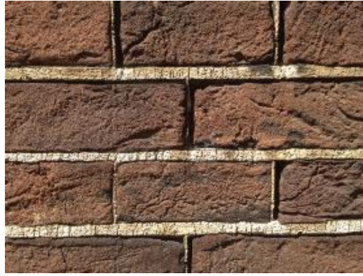
Figure 14. Cut to shape pointing, with typically very high binder content, showing shrinkage cracks.
