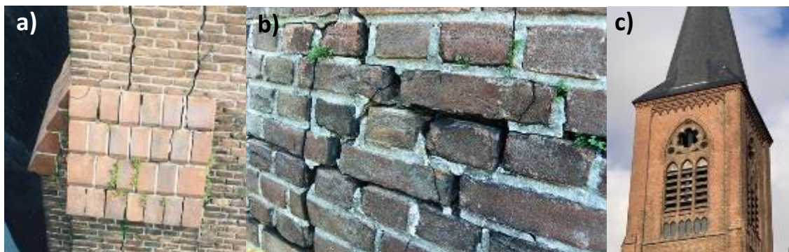
Figure 19. Cracks in masonry, caused by expansion of bedding mortar, deeper in the wall section, due to formation of thaumasite (a); push out of the pointing is a secondary effect (b); situation several years after repair: no recurrence (c).
