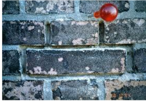
Figure 18. Weak, decayed trass lime re-pointing.
