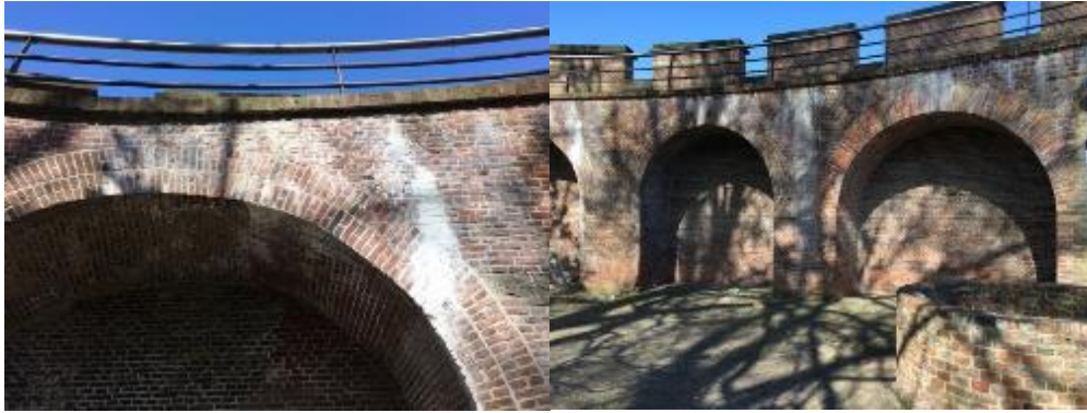
Figure 16. Lime leaching after repair of historic masonry.
