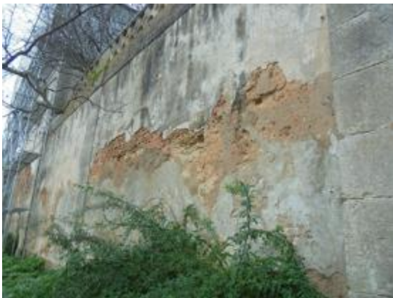
Figure 23. Degradation on the East façade.
