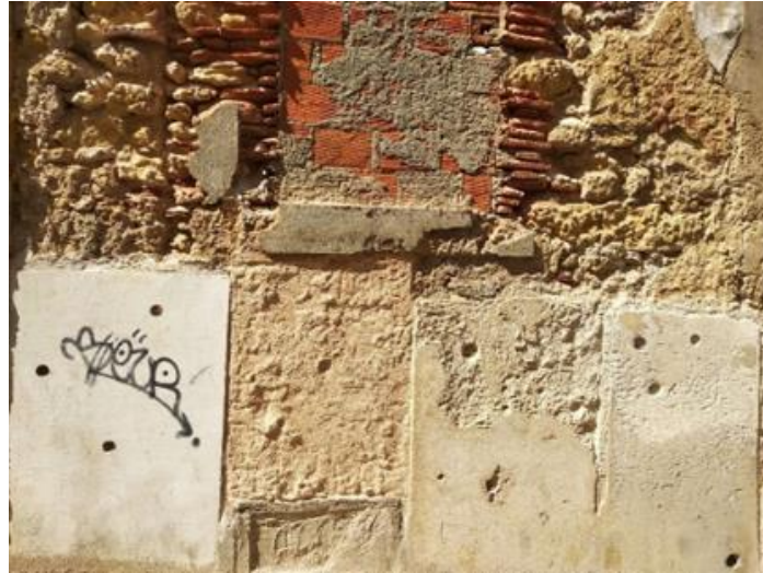
Figure 5. Experimental panels applied on an ancient wall in the Historic Centre of Palmela (Portugal), 12 years after application: second from the left is air lime + MK and third from the left is has air lime as only binder.
