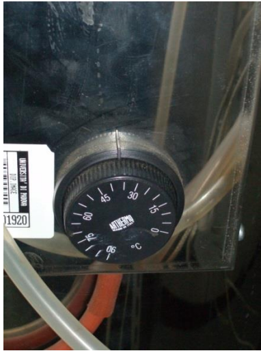
Figure II.5 Picture of a thermo-regulator from an insulation system.
