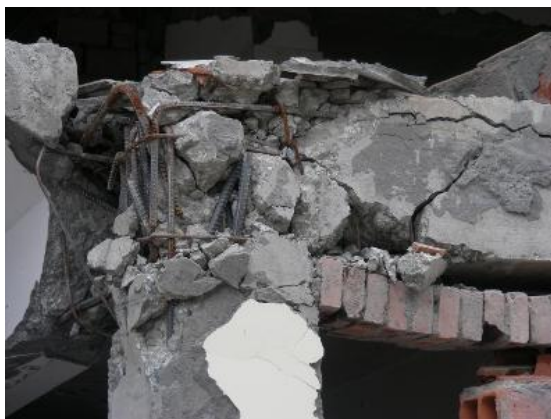
Figura 2.11 Rotura do nó (China, Wenchuan 2008) [NEES-Anchor]
