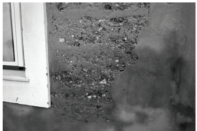
Figs. 2a, b and c Rammed earth market house in S. Luís, Odemira, Portugal, source: M. Idália Gomes (a) market house in 2004, (b) and (c) market house in 2013 with detail of the repair
