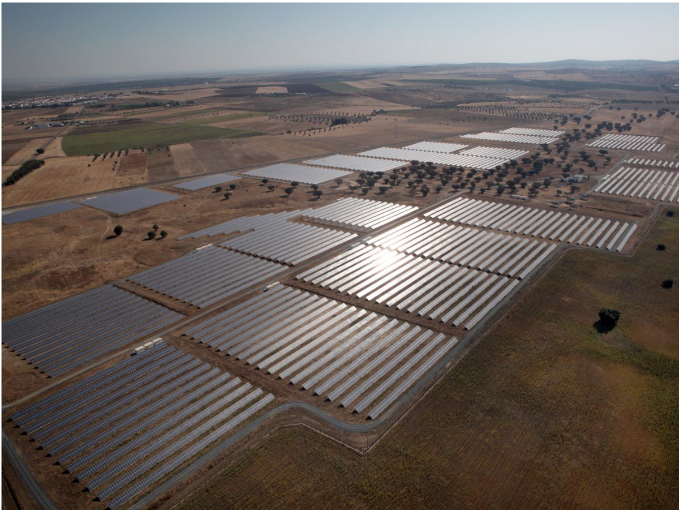
Figure 4 – Photovoltaic power plant in Ferreira do Alentejo, Lower Alentejo (TOTAL Eren, w2022)
