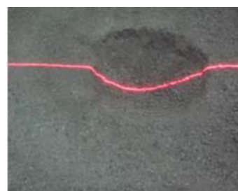
Figure 3. LED light band in pothole.
