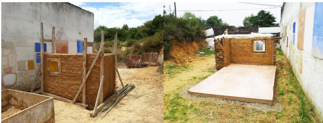
Fig. 4. Reedcob experimental wall of prototype 2 including corner: (a) facing South with provisional formwork; (b) facing North with formwork already removed.
