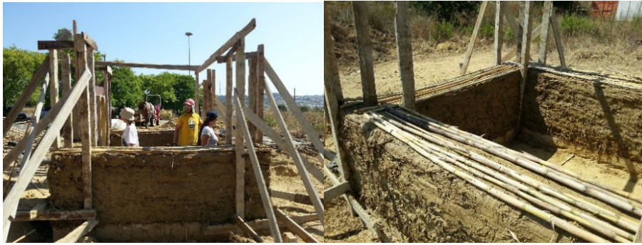
Fig. 6. Reedcob cellule of prototype 3 under construction: (a) general view with students building the walls; (b) detail of a reed layer on the wall being built.
