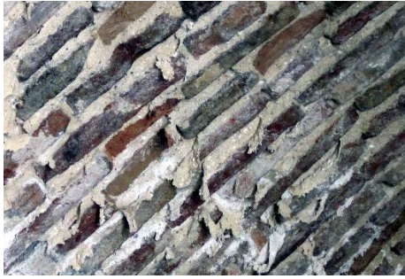
Figure 3 – Example of mortar binder leaching in a building.
