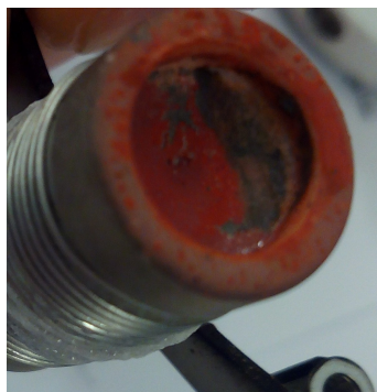
Figure 4.20: Red colouring on the evaporator.
