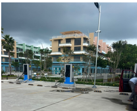
Figure 20: Charging Ports in Phu Quoc (own picture)
