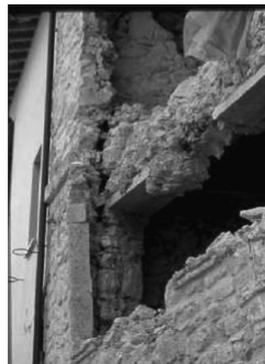
Figure 2.3: Damage detected in a masonry building repaired by introduction of concrete tie beams. Out-of-plane mechanism: separation of leaves. (Courradi et al. , 2008).
