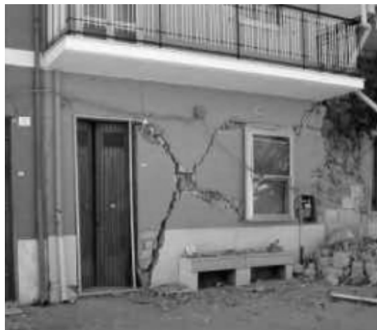
Figure 2.4: In-plane shear failure of the masonry walls (Decanini et al. , 2004).
