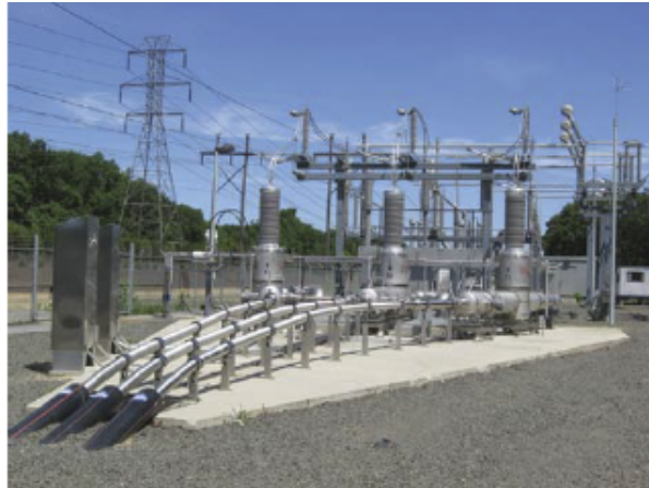
Figure 2.17: Termination of the superconducting cables manufactured by Nexans and AMSC (Rogalla & Kes, 2011).
