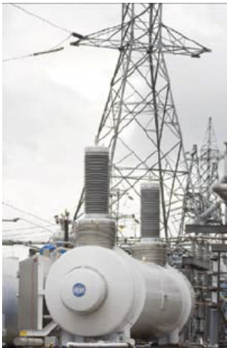
(a) Siemens/Nexans/AMSC resistive SFCL.
