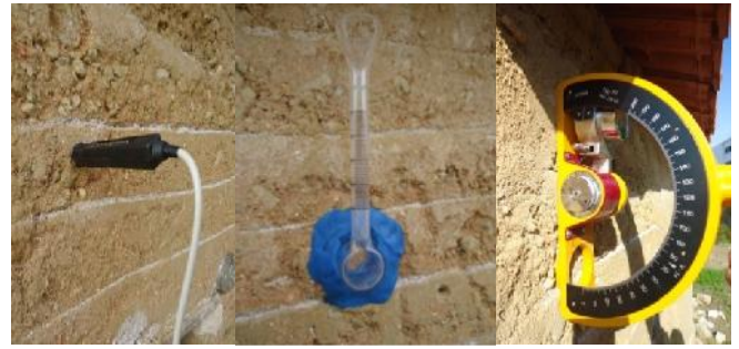
Figure 1. Rammed earth wall being tested for thermal conductivity, water absorption and hardness by sclerometer.
