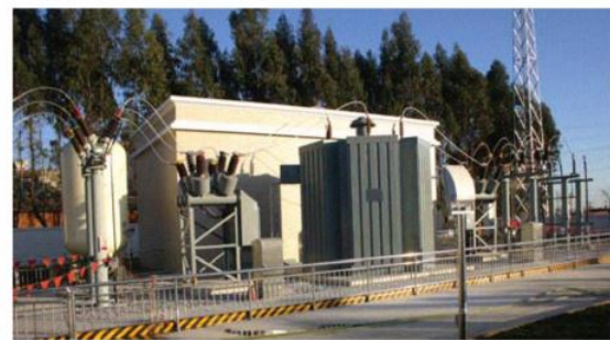
(b) Photograph of the installation of the SIC-SFCL at Puji Substation [32]
