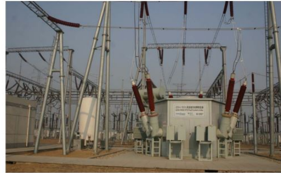
(b) Photograph of the installation of the SIC-SFCL at Shigezhuang substation of Tiang, China [34]
