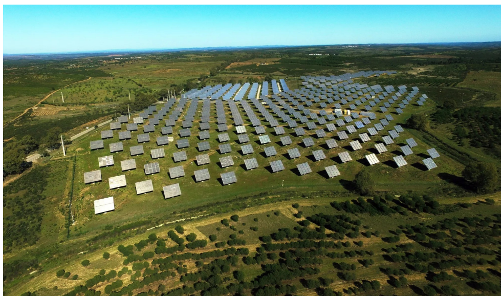
Figure 6.1: Solar Panel farm where large-scale pilot number nine takes place, located in Alcoutim. Taken from “ENERCOUTIM webpage”, 2023
