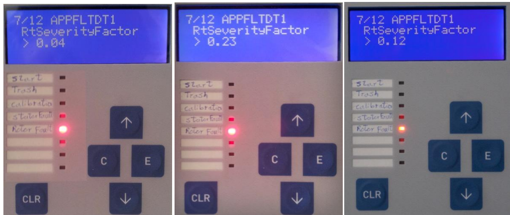
Figure 6.43 – HMI of the TPU with the indication of a rotor fault
