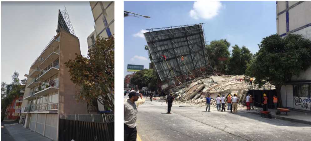
Figure 1.3: Collapse of a building with flat slabs in Mexico City during the 2017 Puebla-Morelos earthquake. Photo before (left) and after (right) the earthquake. (Images collected by Galvis et al. 2017 from Google Street View and media reports)
