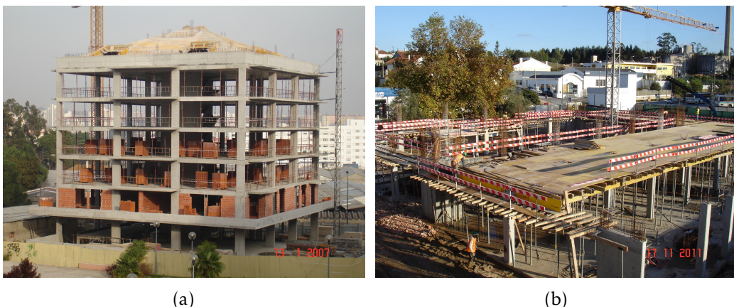
Figure 1.1: Examples of buildings with flat slabs in earthquake prone zones in Portugal (photos courtesy of Válder Lúcio)
