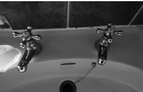
Fig. 12 - Typical separate taps Source: Author's picture, Nottingham [15/02/2015]
