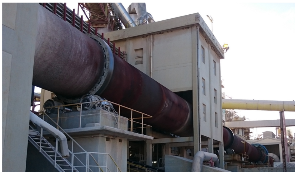
Figure 3. Picture of the rotary lime kiln object of this study (courtesy of The Navigator Company).
