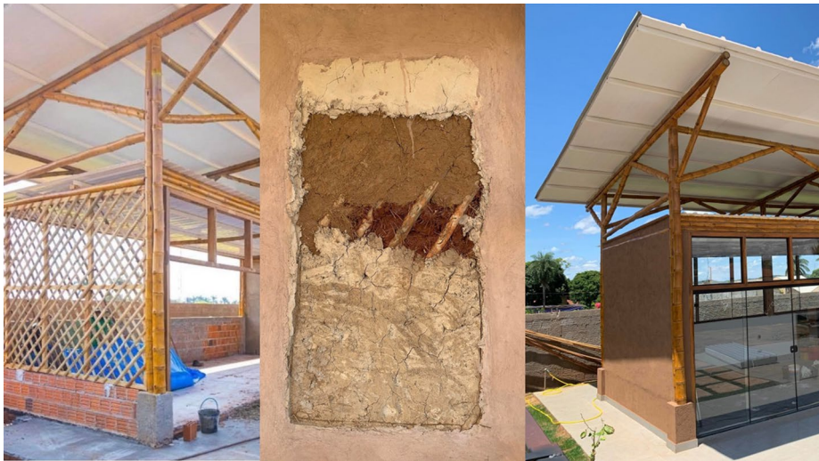
Fig. 1 Residential project with taipa de mão walls. In the images it is possible to see the brick elevation structure, the primary horizontal and vertical wooden structure, and the secondary structure made of bamboo in the transversal direction. The variation between the internal and external layers of the wall. Project by Karin Schwambach, Bonito, Brazil
