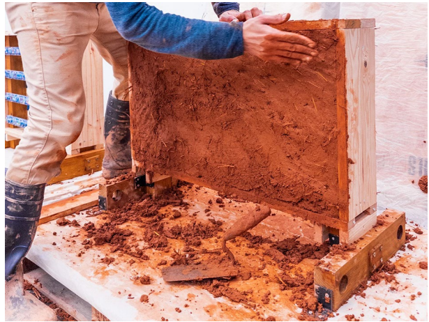
Fig. 8 Earth plastering process of the PA4 prototype. Prototype dimension 800 \times 450 \times 160 millimeters, composed of two panels measuring 800 \times 450 \times 20 millimeters each
