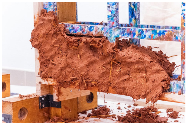
Fig. 6 Application of earth plaster on the PA4 Prototype, consisting of two prefabricated lattices in recycled high-density polyethylene with dimensions 800 \times 450 \times 20 millimeters each panel
