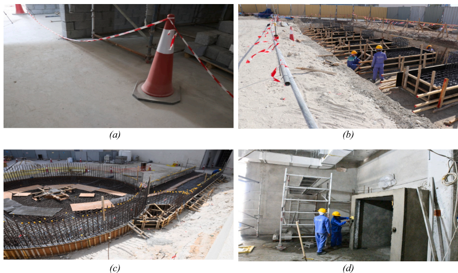
Fig. 7. Selected images from the collected dataset, showing (a) corridor safety barriers, (b) foundation formwork and rebar installation, (c) curved wall construction preparation, and (d) HVAC and electrical system installation.
