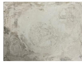
Figure 27 Corrosion of plaster after scrapping the accumulated salts. (©Nour Ali).
