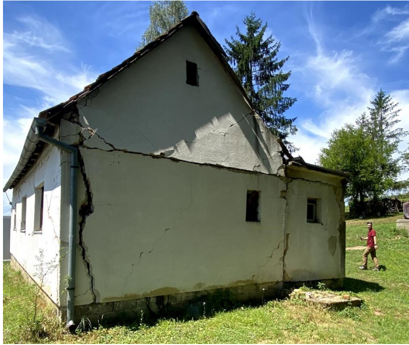
Figure 3.25 - Failure out-of-plane mechanism caused by the existence of a rigid floor.
