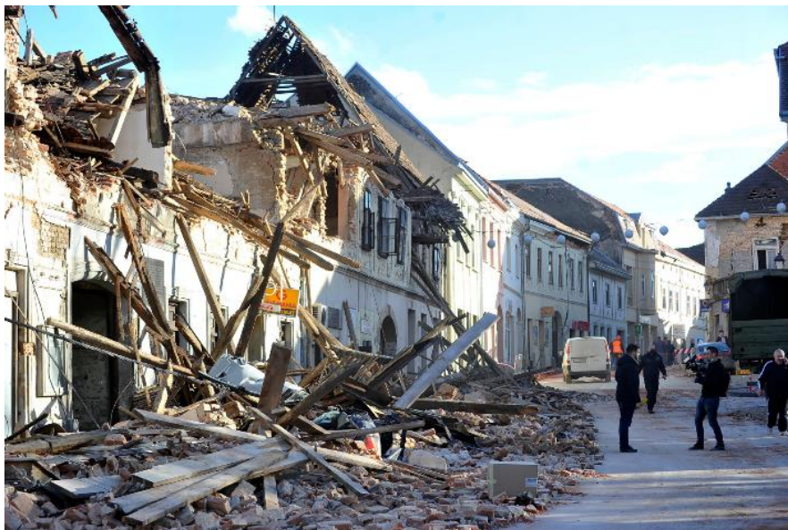
Figure 2.1 - Damaged and collapsed masonry buildings: collapsed buildings after the 2020 earthquake in Petrinja, Croatia (Reuters, 2020).
