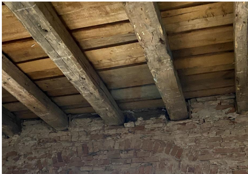
Figure 3.1 - Timber floor of a school building in Zagreb Croatia, this image belongs to the EESD repository.
