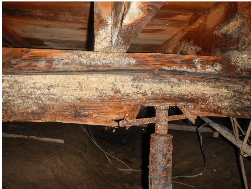
Figure 3.9 - Timber floor with biological deterioration and ageing.
