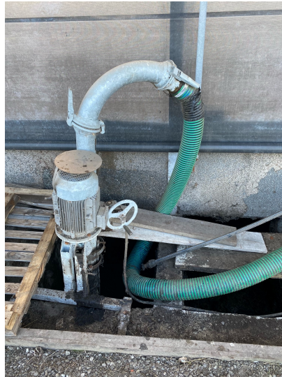
Figure 2.6: Manure Cellar Pump.
