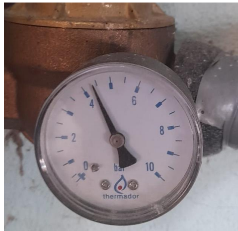
Figure 5-15. Cooling water provided by the local plumbing system with 4.5 bar at room temperature.
