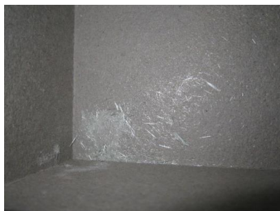
Figure V.13 – Detail of card tray contaminated with asbestos particles.
