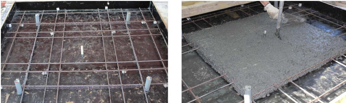
Figure 3 – Steel net used as a formwork for the HSC region (left), casting phase of the HSC region (right).
