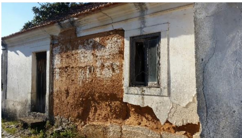
Figure 8. Rammed earth with several basal erosion (inspected building 20)
