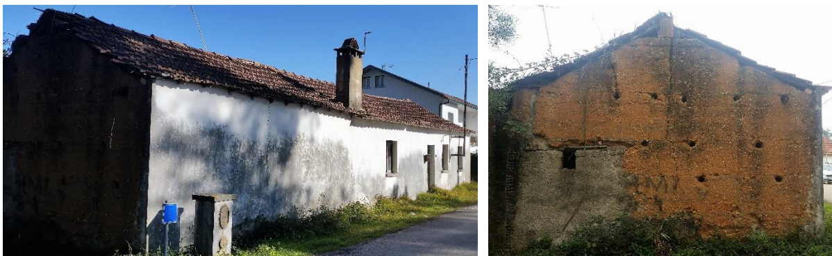
Figure 12. Rammed earth dwelling from Pombal, Portugal (inspected building 29)
