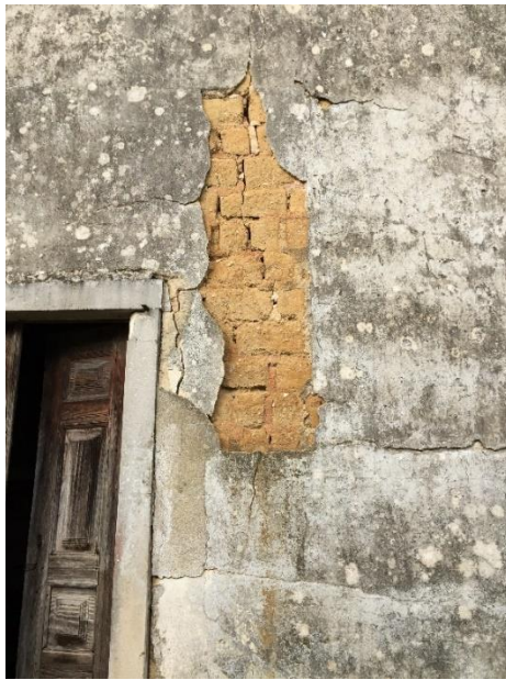
Figure 7. Traditional dwelling repaired with cementitious-based render showing detachment after damaging the masonry surface (inspected building 17 – East facade)
